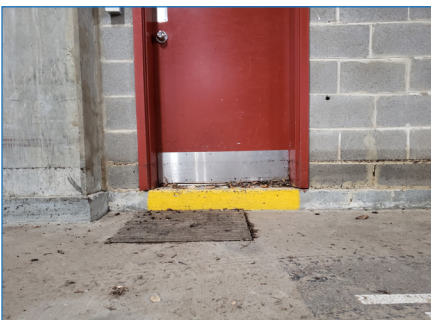
Showing line of floodwater in HQ garage.
