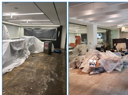
Less than six hours after the rains stopped, clean up well underway!
